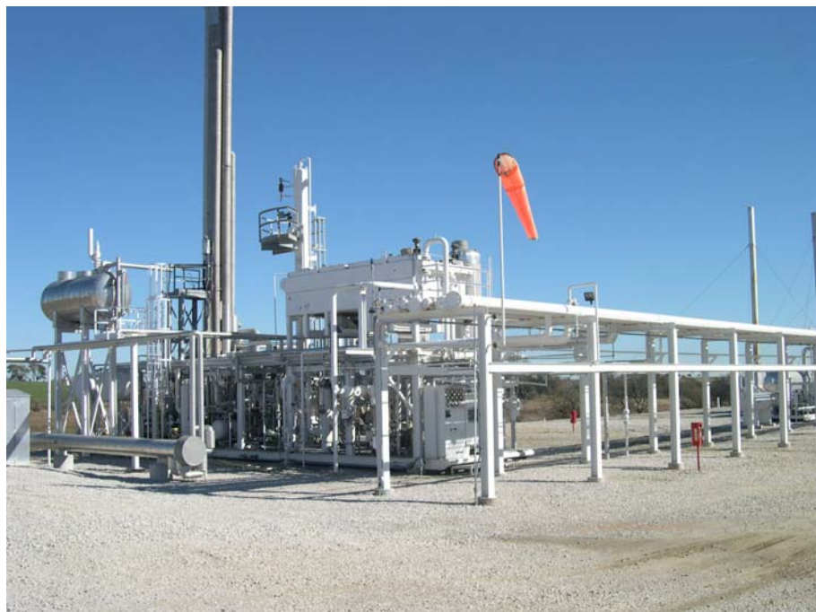
Figure 3. Small Natural Gas Processing Plant (Denton County, Texas).
