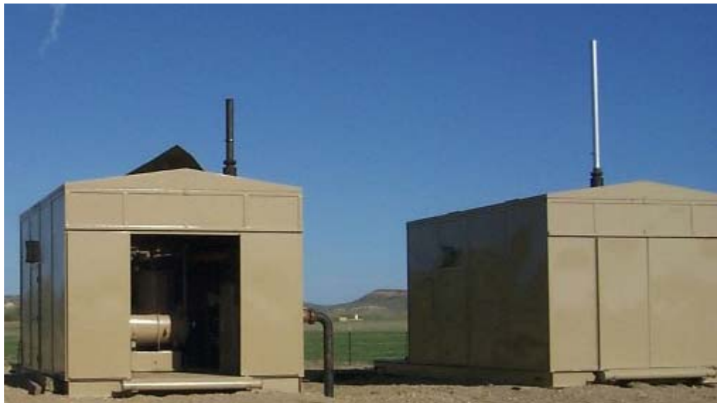
Figure 4. Small Compressor Station (Montana).
