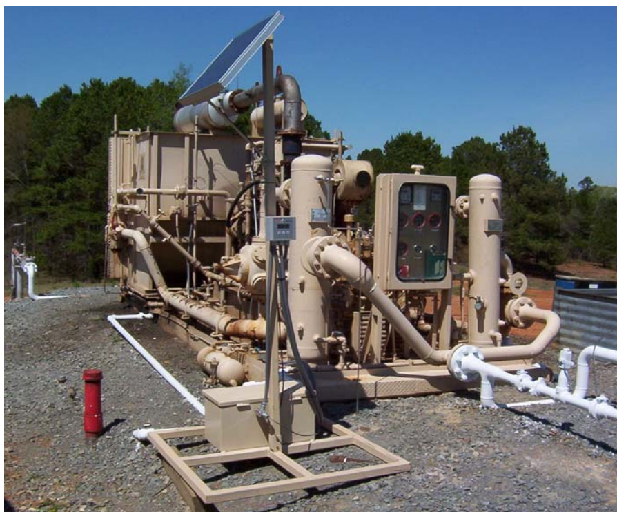
Figure 2-3. Wellhead compressor engine.
